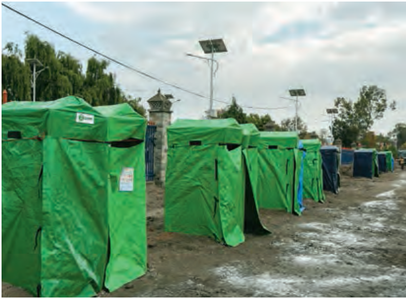
⤴ Oxfam quickly constructs 20 pit toilets to serve 5000 people at the Tundikhel camp
