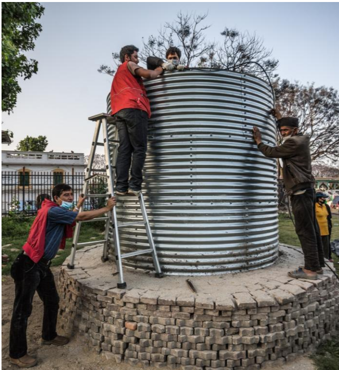
Oxfam staff and volunteers construct an 11,000 litre water tank at Tundikhel IDP camp. Oxfam is providing water to 15,000 people here. Photo: Pablo Tosco / Oxfam
